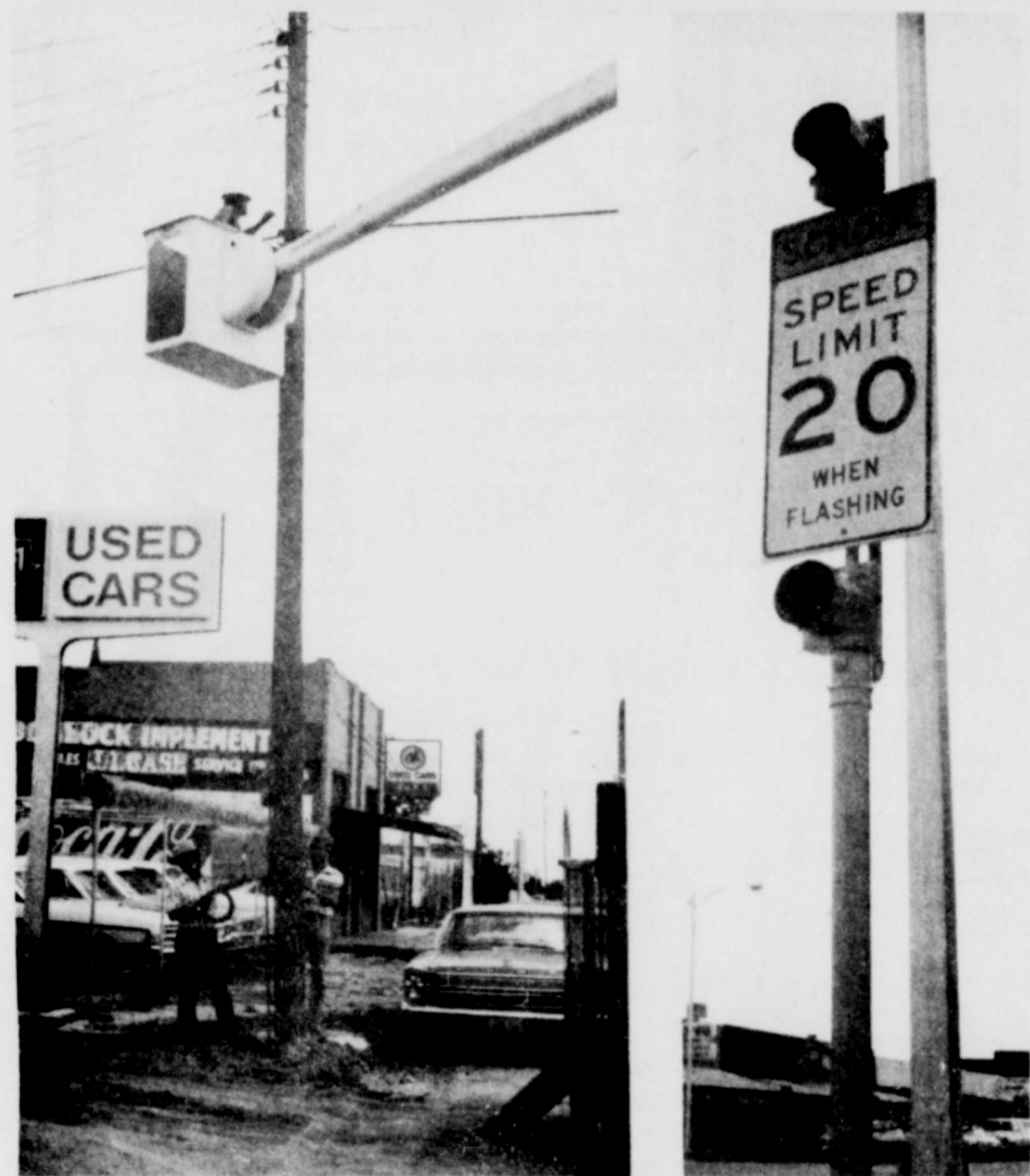
FINAL STEPS--in the installation of the new traffic signs which will help protect school children crossing Avenue D, were completed early this week as the new signals were connected to power sources. (left). The lights, furnished by the state department of highways and public transportation, will be in service, warning motorists to slow to a speed of 20 mph during school hours when the fall term begins August 20. (right photo). (staff photos)
