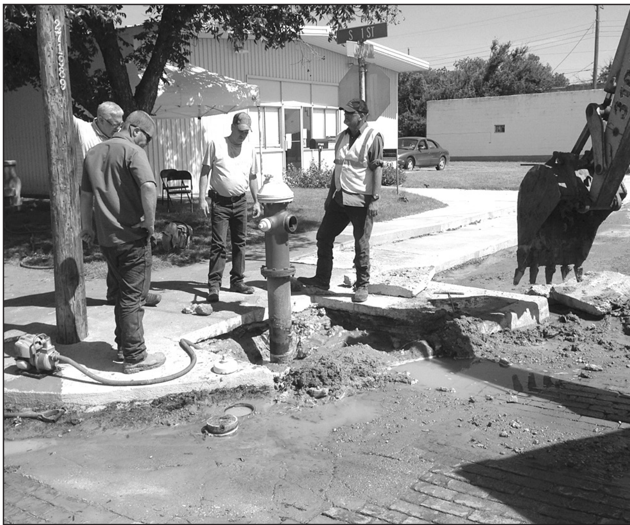
IT'S ABOUT THE WATER —City employees, l-r, Joseph Payne, Brandon Anderson, Matthew Duran and Gerald Stanford discuss the plan to repair a leaking fire plug at South 1st Street and Avenue D. Hot weather, causing the ground to shift, and aging infrastructure all contribute to water leaks. The City works to deal with the problem while complying with the Stage 3 Drought Contingency Plan.
