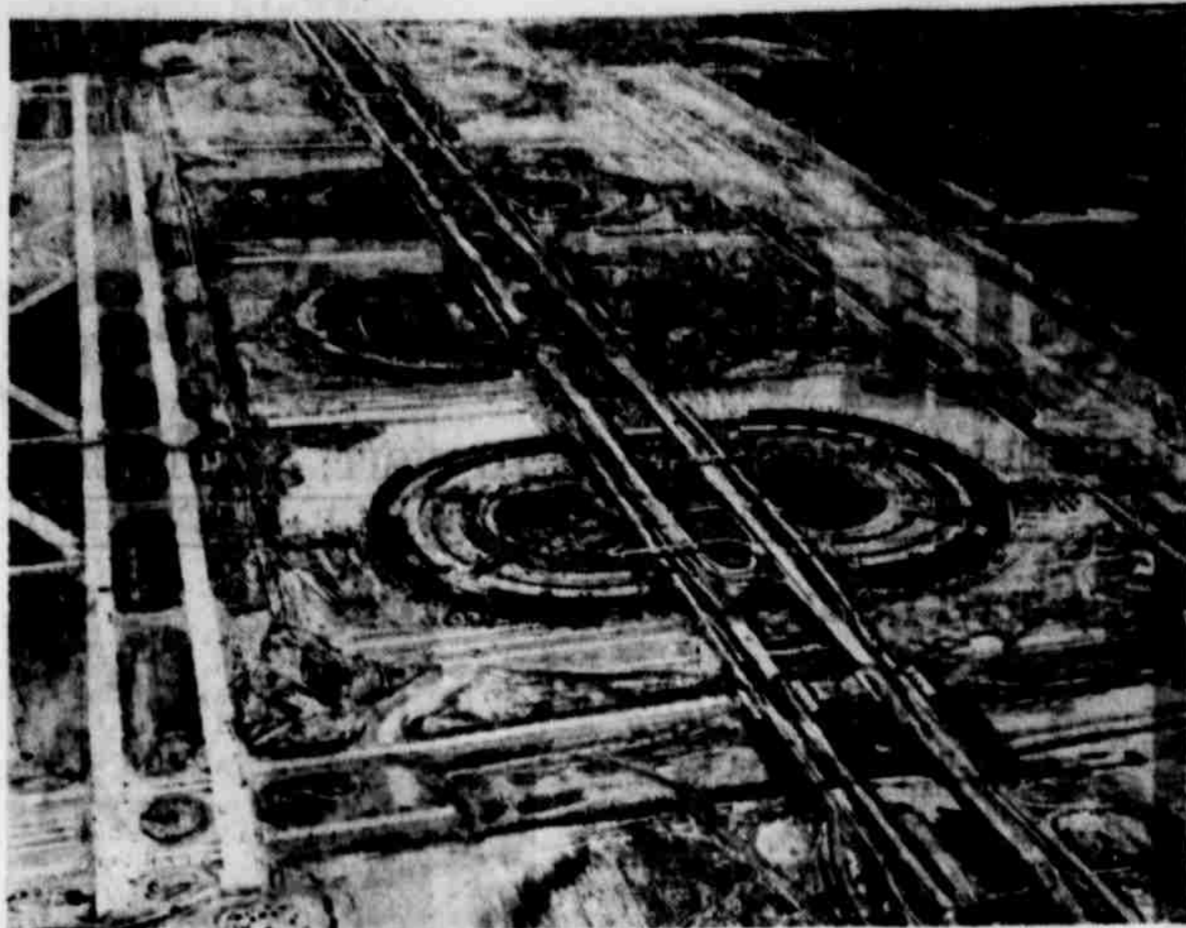
TEXAS-SIZE SUPERPORT —This aerial view of the new Dallas/Fort Worth Airport shows construction progress on the giant superport scheduled for opening in early fall, 1973. Conveniently located 17 miles from both Dallas and Fort Worth, the new airport is designed with the passenger in mind. Drive to gate boarding, close-in parking and simplified terminal procedures are only a few of the ultra modern features designed into the unique facility.
