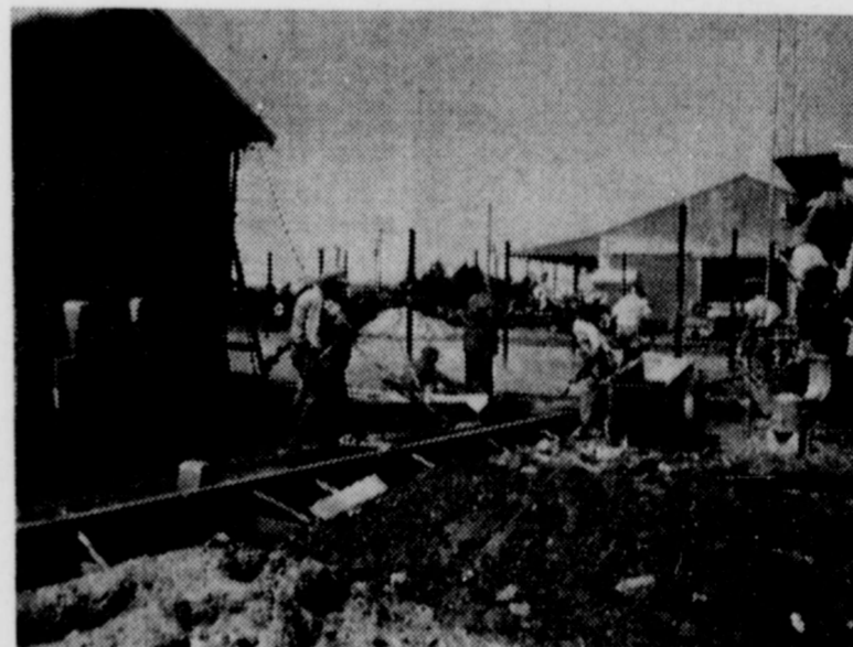
LARGE ADDITION — This picture shows workmen busy constructing a large masonry-type addition at Joe Thompson Implement Co. The new portion, when completed, will house the John Deere parts department and the company's offices.
