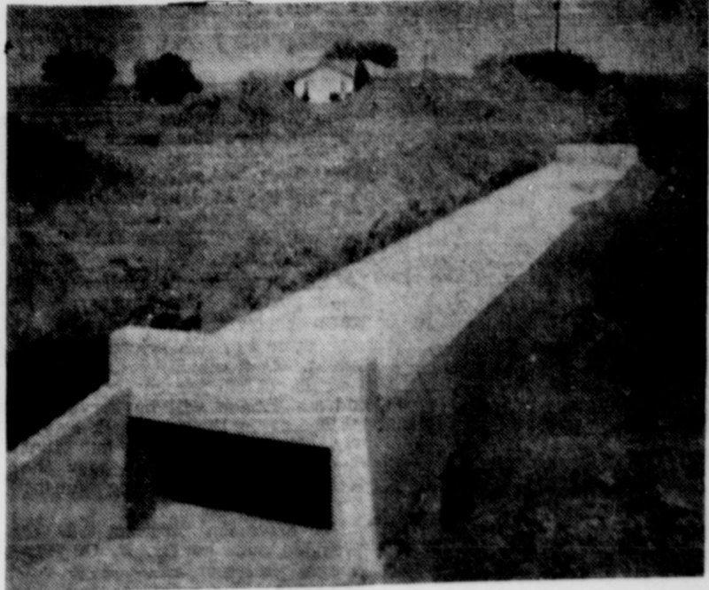
NEW ON U. S. HIGHWAY 87 —Two new lanes are to be built west of, and parallel to, the present lanes of U. S. Highway 87 to make a four-lane divided highway between Abernathy and Hale Center. The culvert pictured above is one of several being built for the two new lanes. Top right in the photo is the culvert for the present lanes of the highway. The M. D. Evans home, about a mile north of Abernathy, is in the background.—(Review Photo)
