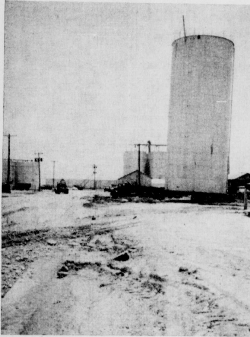
TANK MOVED—This picture was made last week while movers were taking the water storage tank off the railroad right-of-way and relocating it about a quarter of a mile south on the Plains Grain Co. property.
