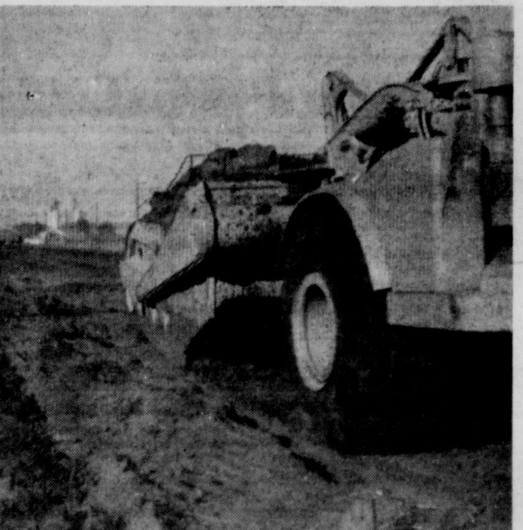
THE RIG shown at the right in this picture is one of several earth-moving units that will dig the underpass to carry through traffic on the new freeway being built through Abernathy. Several hundred thousand tons (one estimate said 500,000 tons) of yards of dirt will be moved to build the underpass. Main Street traffic in the center of town will be on ground level and the freeway traffic will be in the underpass under Main Street. This picture is looking north from Main Street along the wide, cleared right-of-way for the freeway and service streets to be constructed on both sides. Dirt from the underpass construction will be used in bases for overpasses to be built for freeway traffic on the south and north ends of town — (Staff Photo)
