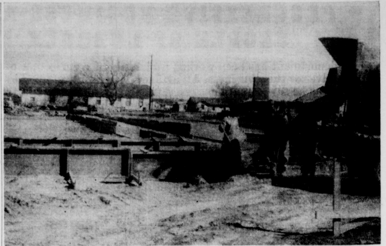
CONSTRUCTION WORK of the new buildings on the Abernathy school campus is progressing on schedule, according to reports. In the above photo construction workers are shown pouring concrete at the southwest corner of what will be the new Primary building. A. P. Kasch & Sons of Big Spring is the contracting company. (Photo By Boyd Mitchell)
