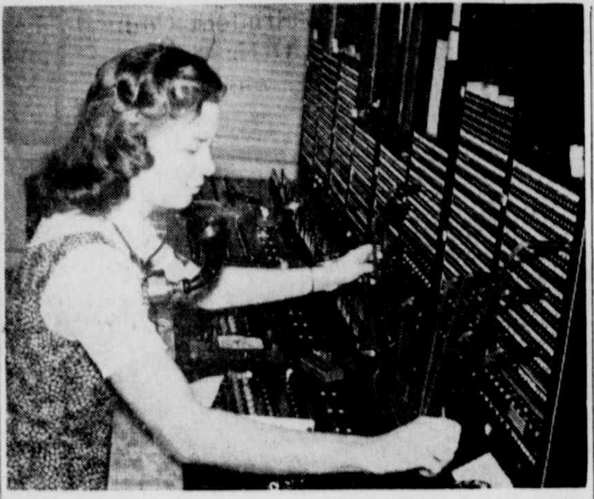
MRS. TRAVIS HOWARD was Abernathy's last telephone switchboard operator. Mrs. Howard is shown here working the final shift before Abernathy's telephone system was converted to automatic dial. Mrs. Howard went on duty at 10 p. m. Nov. 30, and worked until the dial system was placed into operation at 6 a. m. Dec. 1. —(Staff Photo)
