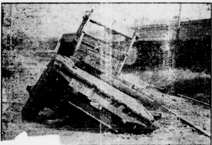
Kansas City, Mo.—Laden with an overloaded tonnage of steel, here is what happened to the highway of an outer-belt road leading into Kansas City. The right rear wheel cannot be seen as it is completely submerged in the concrete slab. So many highway accidents have occurred in this state and the need for data which may be used as a basis for determining the special road costs incurred by trucks is so great that state highway departments are now conducting surveys in several states to determine a fair charge against the trucks for the use of highways. While thousands of motor trucks daily bring about destruction of highways shown in the above illustration, it is pointed out that pleasure cars and light farm and delivery trucks stand an unjustifiable share of costs of highway upkeep.
