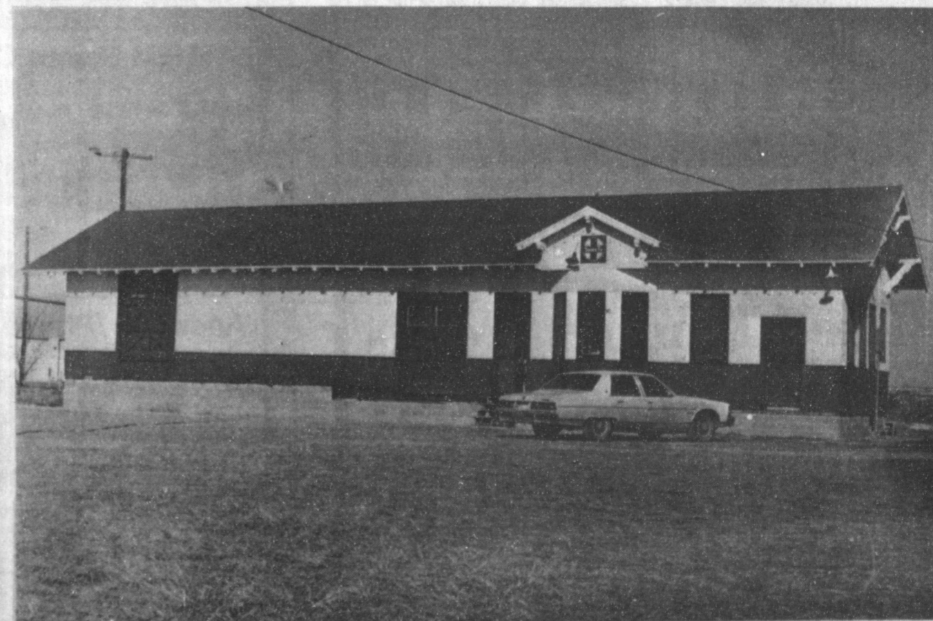
WINTER RENOVATION CONTINUES --Even though it is wintertime, renovation is continuing on the old Santa Fe Depot, which is in its permanent location at the Ranching Heritage Center. When completed, the depot will become a senior citizen center. Santa Fe Railway donated the depot to the Muleshoe Heritage Foundation, who moved it last spring to its new location.
