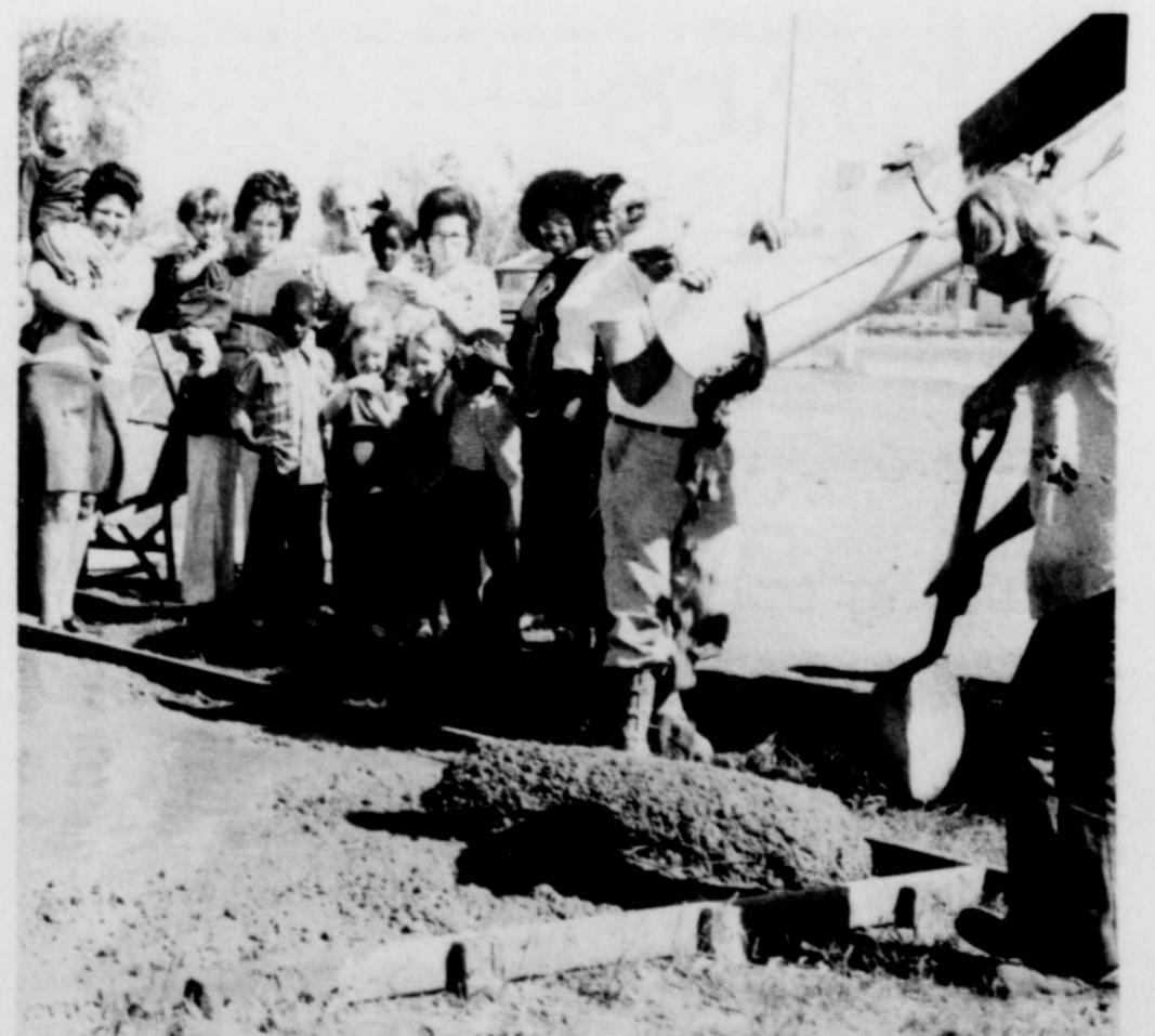
STORAGE SHED SLAB --Theta Epsilon Sorority, with the volunteer help of some of the American Legion Post 264 members, laid a concrete slab for the erection and installation of a storage shed for the Burkburnett Day Care Center Monday. Pictured with several of the day care children are Helen Locklin
