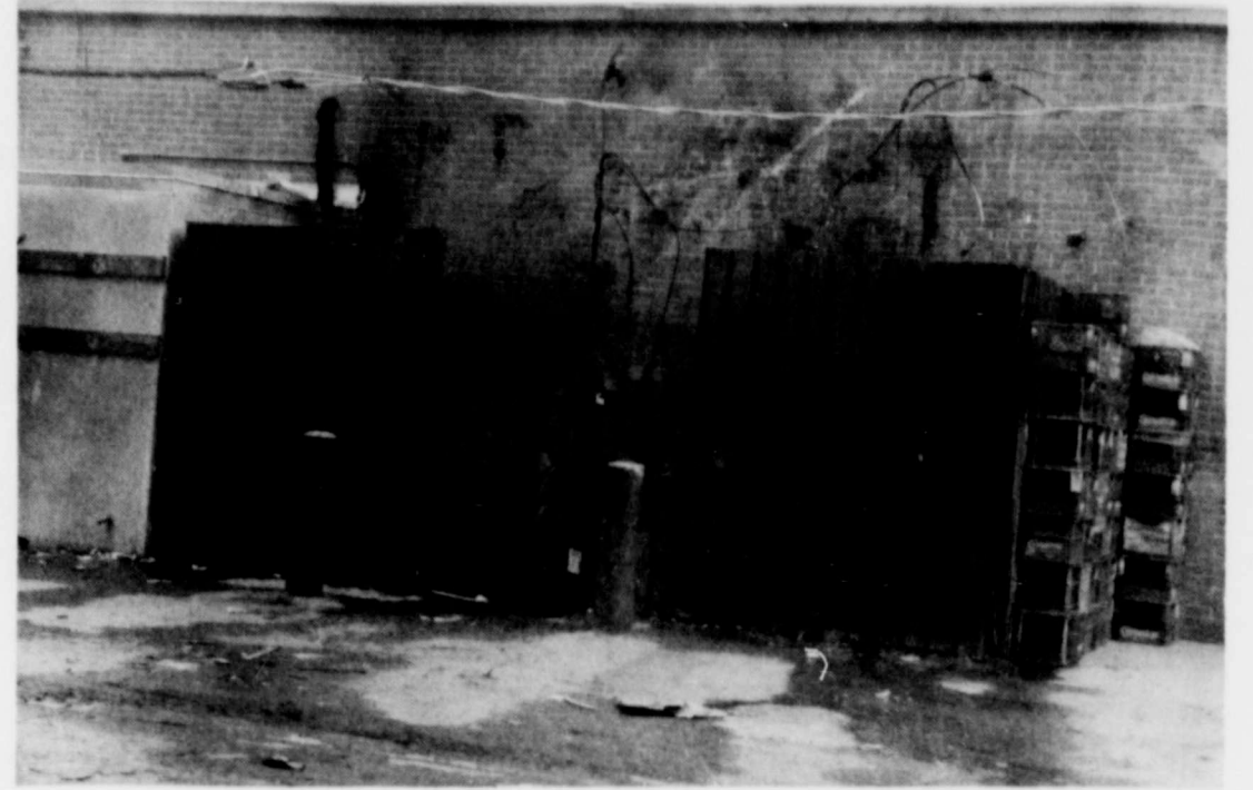
Burk's Parker Plaza Shopping Center lost electrical power last Saturday morning for a short period of time when a fire broke out in the trash container behind Piggly Wiggly. The flames burned the electrical input to the center located just above the container. Electricians quickly repaired the wiring and restored power to the center within minutes after the blaze. Burned wires are seen dangling behind the new repairs.
