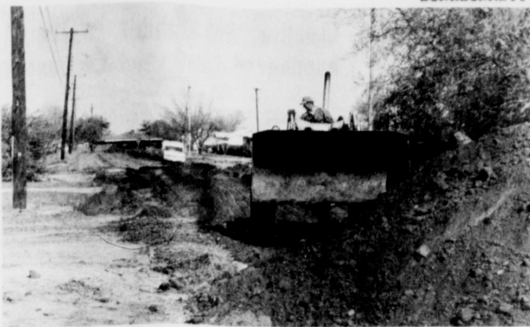
Burkburnett's Revenue Sharing Funds are shown hard at work in this photo of Tidal Street. The street is being completely reworked and represents only one revenue sharing money expenditure. Property owners will be assessed $1.75 per front foot for the curb and gutter and revenue money will take care of the rest. The total cost of the project is $43,000.
