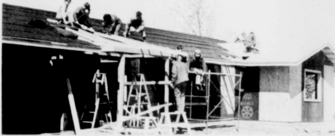
The Building Trades Class shows steady progress on the house they are constructing on Sycamore Street under the supervision of Mr. David Breuer. The Park High School students have constructed the house from the floor up and will sell the finished product.
