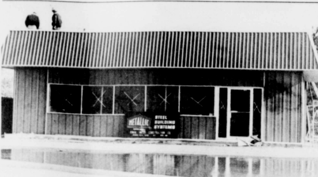
Good progress can be seen at Bills Auto Parts, 903 Sheppard Road, in Burk. The all new metal building has gone up in two weeks and will house a bigger, better and more modern Bills Auto Parts in the near future.
