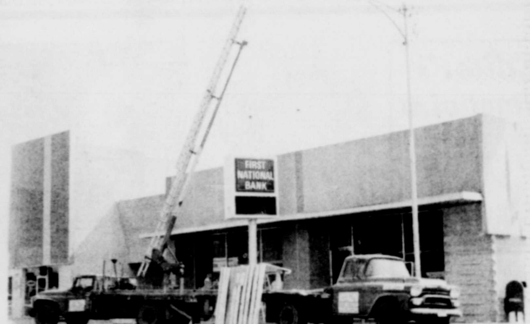
UP GOES NEW CLOCK --Workman worked most of last Wednesday installing the new Time and Temperature clock for the First National Bank. The new clock is in full operation now and is both attractive and helpful to the downtown area.
