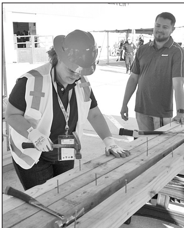
NAIL DRIVING —Rochester VTC student Joslynn Harris of Benjamin ISD participates in "hands-on" activities at the Construction Day.
