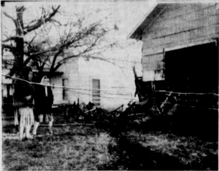
Where S Sgt. Connie Ayatt's car cut through the home of Mrs. Lillie Duke, Thursday, February 1, when it careened out of control at 3:30 a. m. Mrs. Duke, left, and a friend look over the damage.
