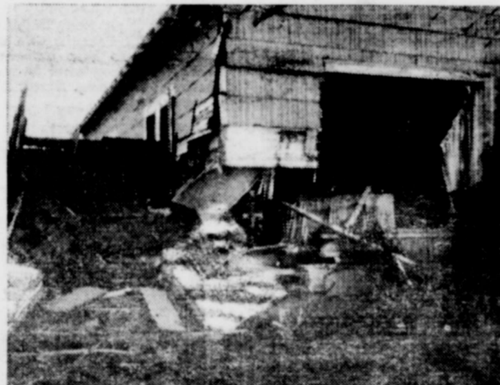
The home of Mrs. Lillie Duke, 114 Avenue D, received extensive damage when struck by a car, Thursday, February 1, in the early morning hours.
