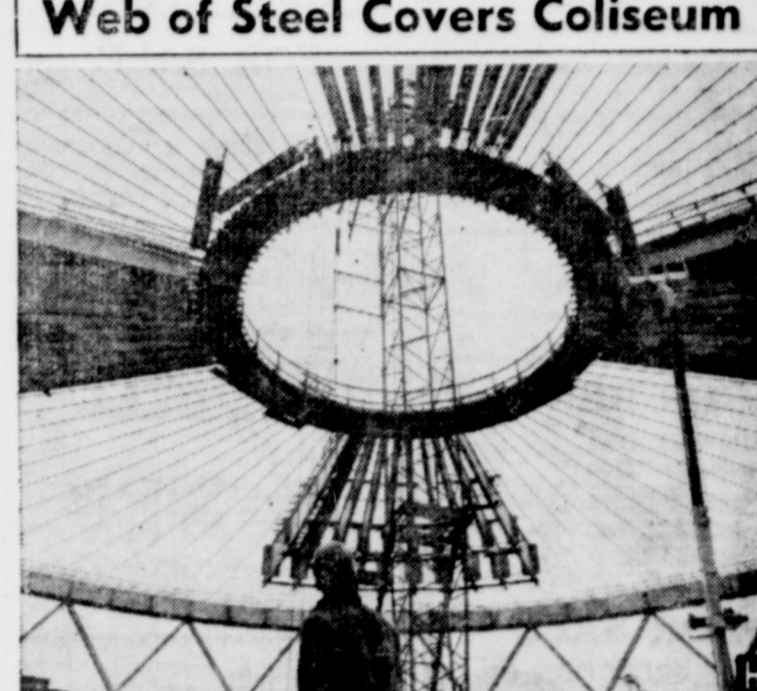
GALVANIZED steel cables spun between inner and outer rings provide the sinewy web for one of the world's largest cable-suspended roofs. California's Oakland Alameda County Coliseum Complex arena roof will span more than 400 feet, providing spectators unobstructed, column-free views throughout the arena.
