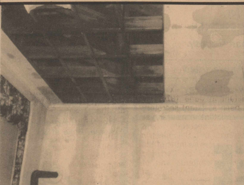
Gee! Do we have problems! This damage and much, much more resulted from wind driven rain at the Kerrick Community Building.
