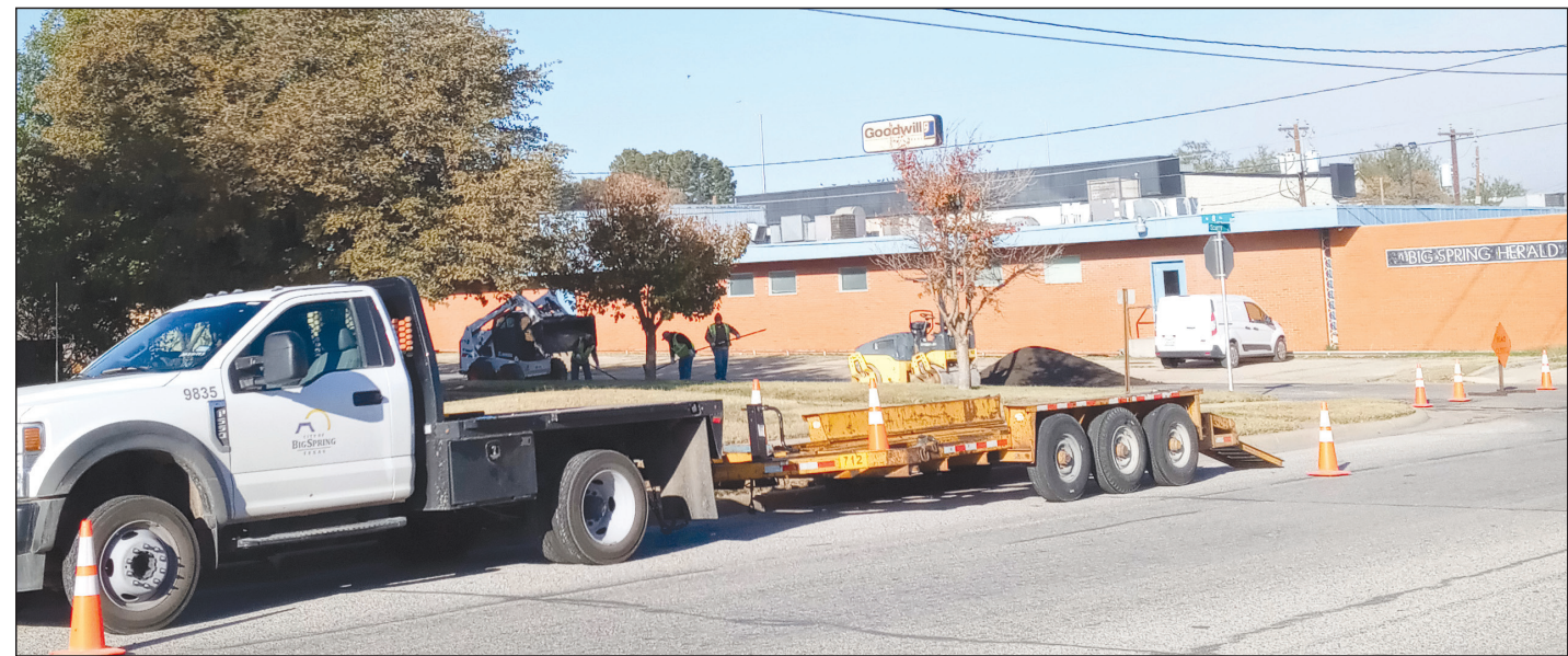
HERALD photo/Andrea Medlin A City of Big Spring road crew was busy pouring asphalt on Eighth Street next to the Big Spring Herald offices Tuesday morning.
