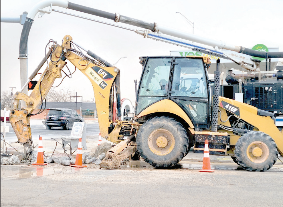
HERALD photo/Roger Cline Shown above, city crews worked to break a hole in the street at the intersection of Gregg and 18th streets Wednesday evening. The work was part of an effort to repair a water main in the area. Work on the water main continued throughout the day Thursday.
