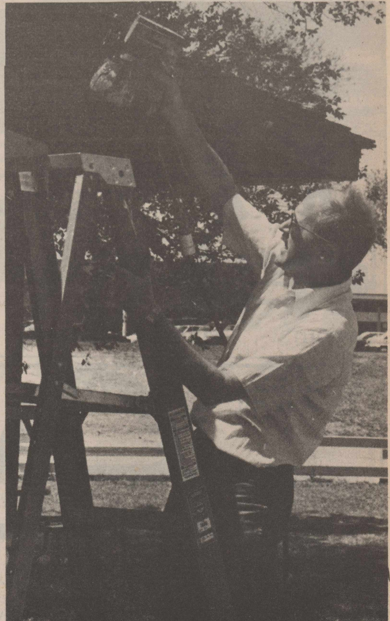
Over 200 volunteers have pitched in to help complete the picnic area renovation project.
