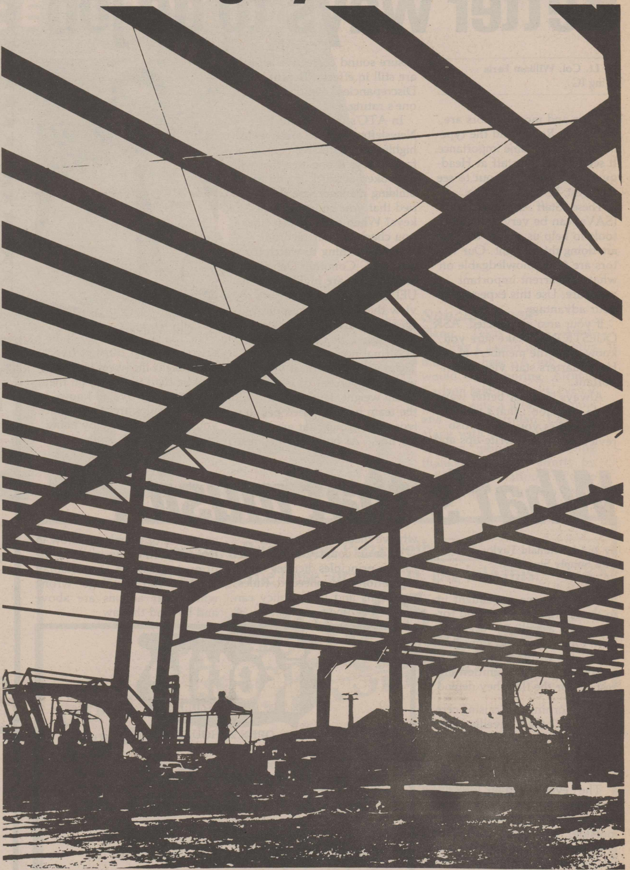
People from the Cooper Construction Company continue work on the new Transportation Complex. Officials said the building should be completed by November this year.
