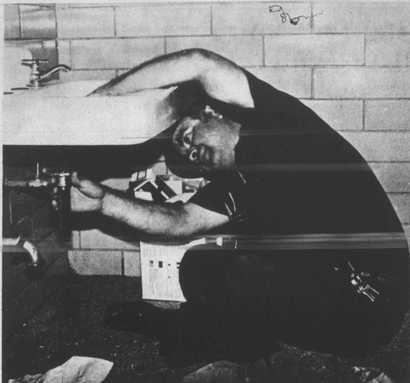
MAINTENANCE — School district maintenance man Jesse Faulkenbery was fixing a sink leak at North Elementary School in preparation for the start of school — part of the extensive maintenance work that goes on each summer. (SDN Staff Photo)
