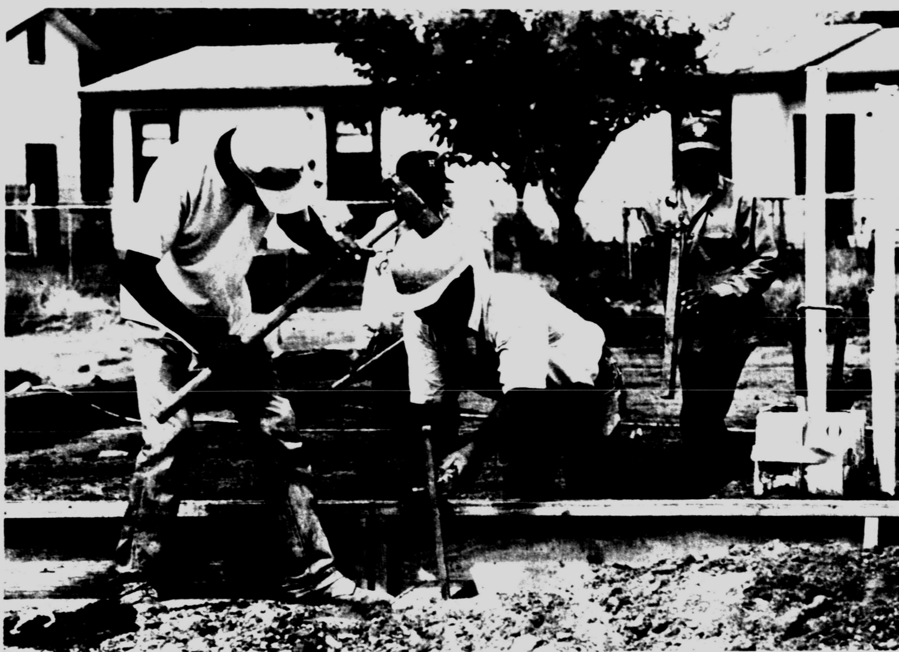
HAMMER DOWN — Rich Galvan was wielding the hammer and Lupe Madrid was holding the stake as Albert Rodriguez, right, and Chico Olivarez of Chico's Concrete worked in the background at the
