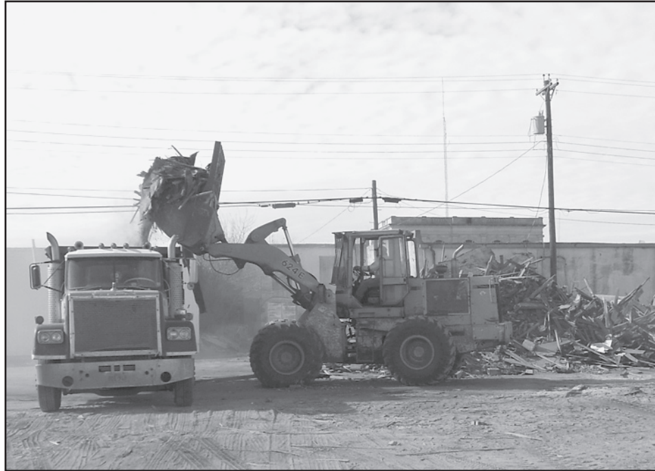
LOT CLEARED —Haskell City employees were busy last week clearing the lot where the old Chrysler building had been demolished.
