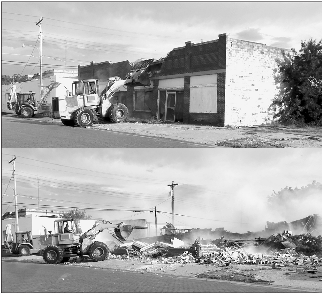
AND THE WALLS CAME TUMBLING DOWN —City of Haskell crews took down the old Chrysler building located across the street from City Hall Wed., June 13. The decision to bring down the building was in the interest of public safety. Currently plans include cleaning up the lot. Possible uses for the area are still being considered, according to City Administrator Brandon Anderson.
