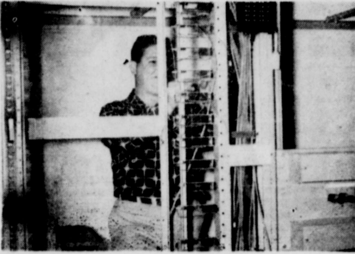
MAIZE OF WIRES—L. C. Camp, who inspects equipment for the Stomberg-Carlson Company of New York, is shown wiring a trunk shelf in the Lenorah exchange of the West-Tex Telephone Co-Operative system. Service on the complete system is expected to be available by May 20, on which date exchanges at Lenorah and West Stanton (Courtney) will have been finished.
