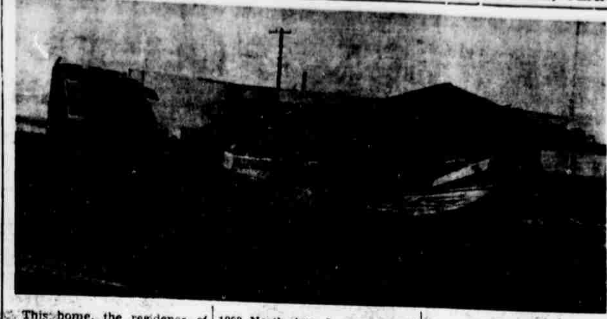
This home, the residence of Mr. and Mrs. Gerald Lytle, 1203 North Ave. L, was one of a dozen or more completely destroyed in the tornado Saturday night.
