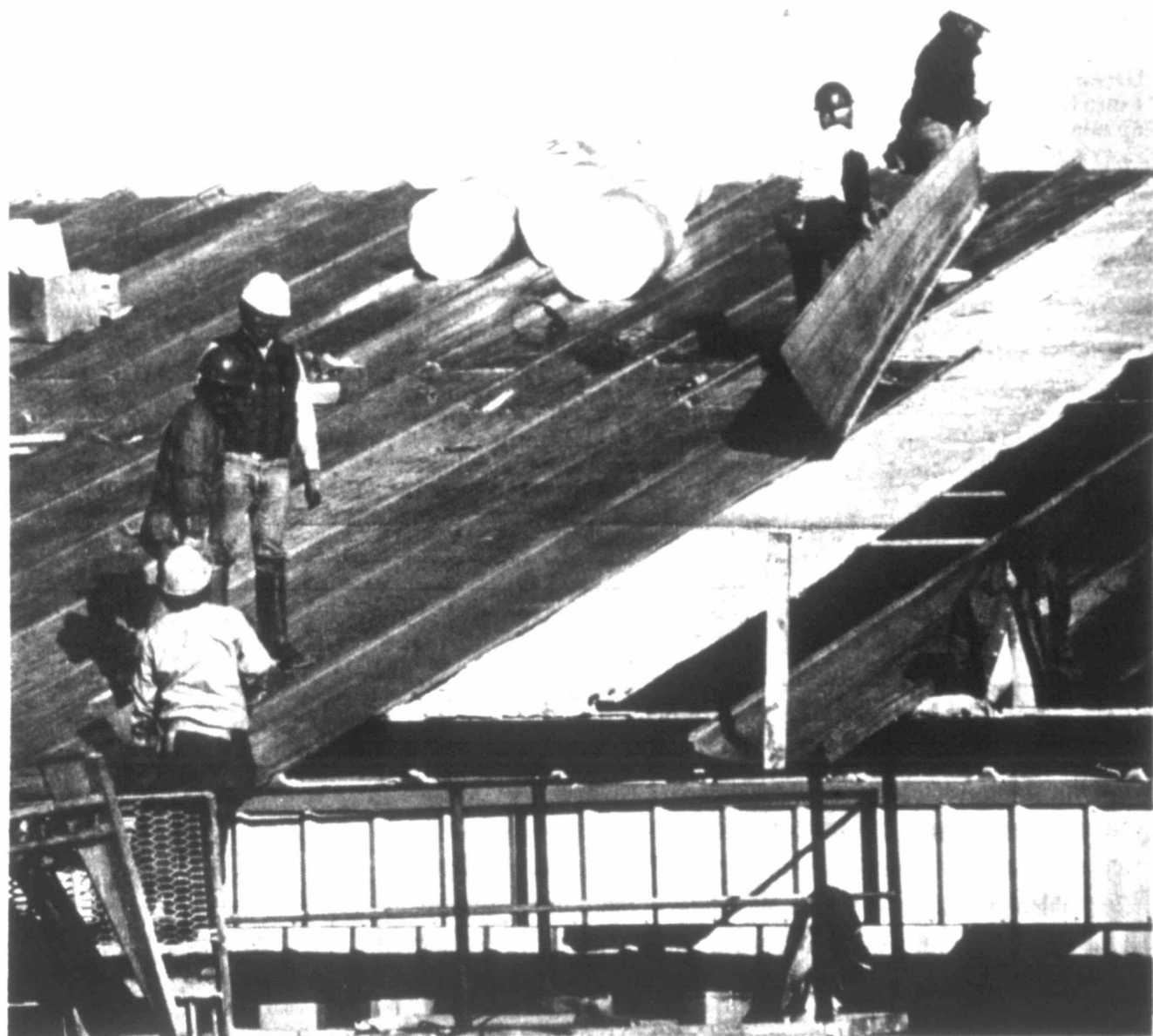
LAYING A ROOF — Workmen at the Texas Department of Corrections Price Daniel Unit construction site five miles northeast of Snyder last week were laying the roof on the complex's educational-vocational building — one of the larger structures at the site. (SDN Staff Photo)
