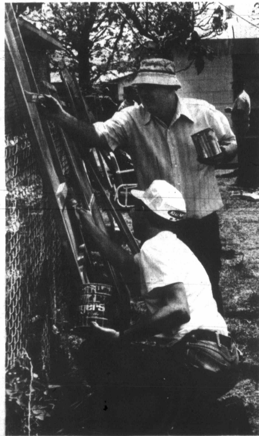
FINISHING TOUCHES — Jerry Vestal and Dewey Farley (standing) put the finishing touches on some windows at a local residence during Saturday's Snyder Neighbors Sharing Day. Over 300 volunteers contributed to the project, which saw repair work being done to more than 20 homes. (SDN Staff Photo)
