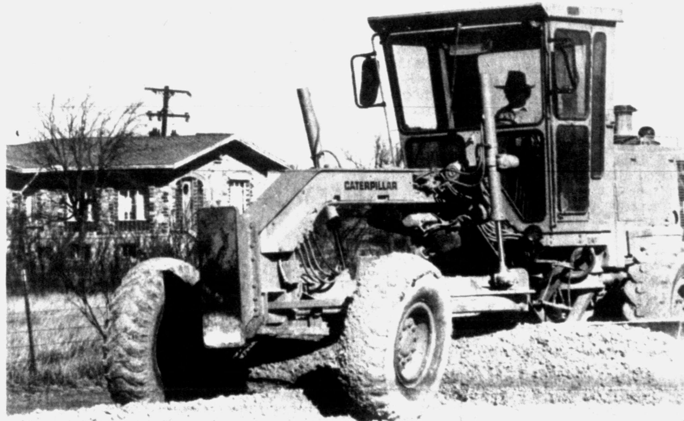
THE NEW CLAIREMONT HWY. — Work on the Clairemont Hwy., which the state highway department is revamping, has reached the 23-mile point northeast of Snyder toward Kent County, where
