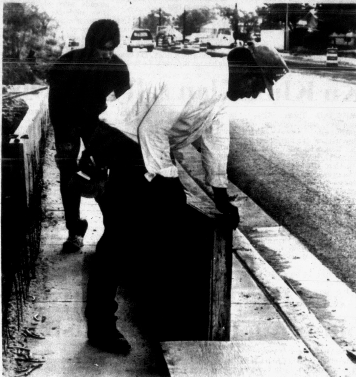
SIDEWALK CONSTRUCTION — Pete Ortiz, front, and Gerald Mireles, straighten forms prior to pouring concrete for sidewalks along 37th St. as work on the street widening project continues. (SDN Staff Photo)
