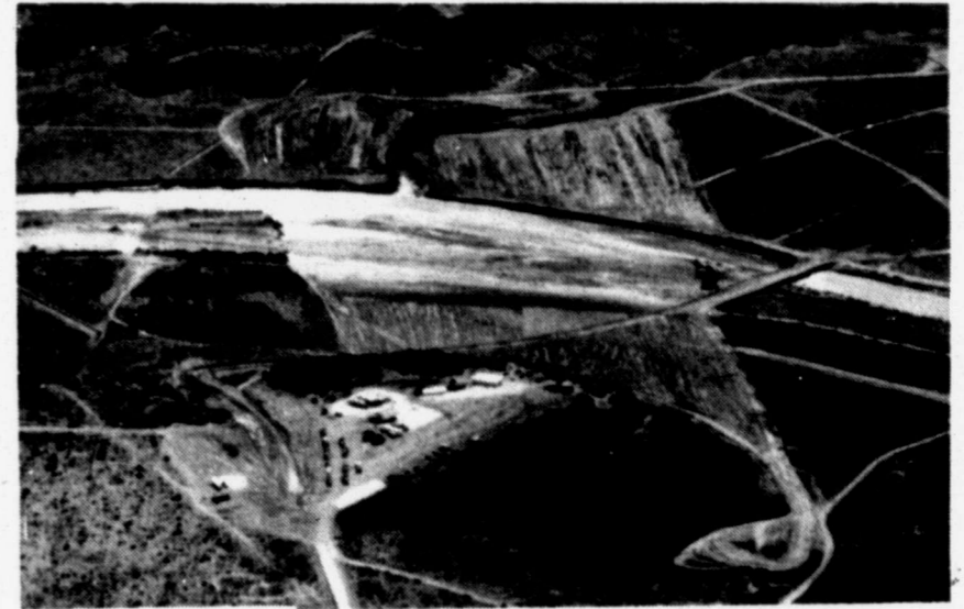
DAM GROUNDBREAKING SET — Dirt work has already begun on the dam for Lubbock's Lake Alan Henry in Garza County, but work becomes official with groundbreaking ceremonies at 11 a.m. Friday. This aerial photograph shows the contractors headquarters (lower center) on the canyon rim. (City of Lubbock Photo)
