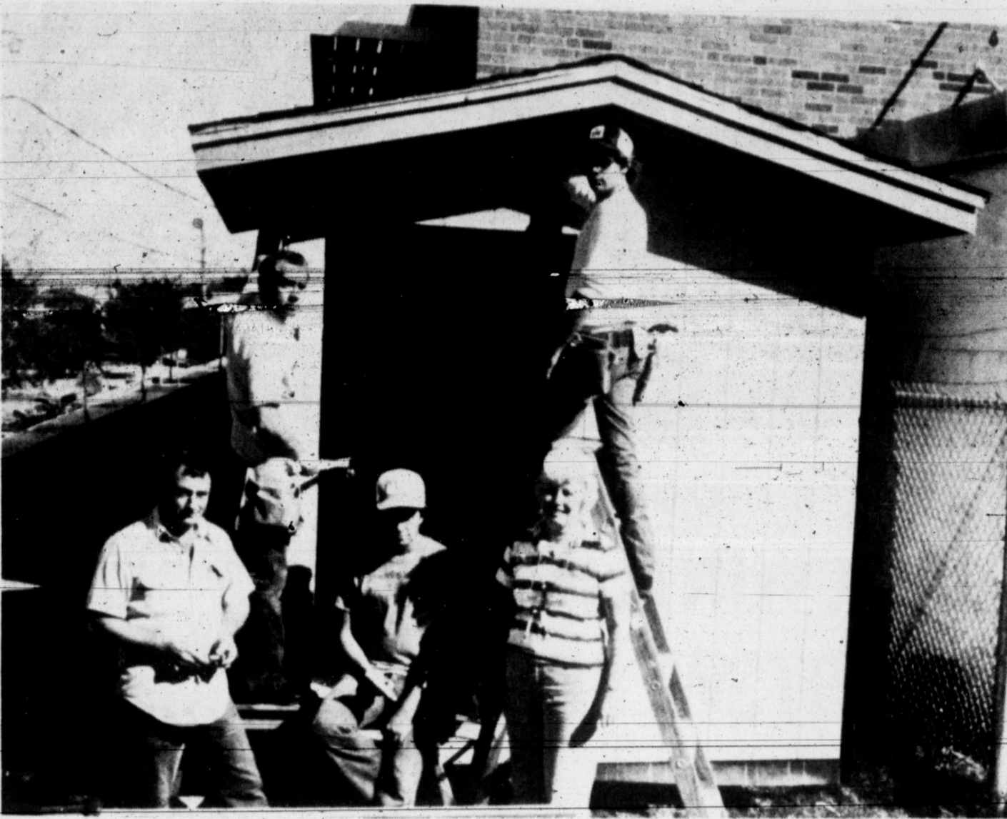
GIVE A HAND —Residential Construction students from Western Texas College, under the guidance of Abel Garcia, instructor, are shown at work on a storage building they are erecting for the Senior Citizens Center. The students are (left to
