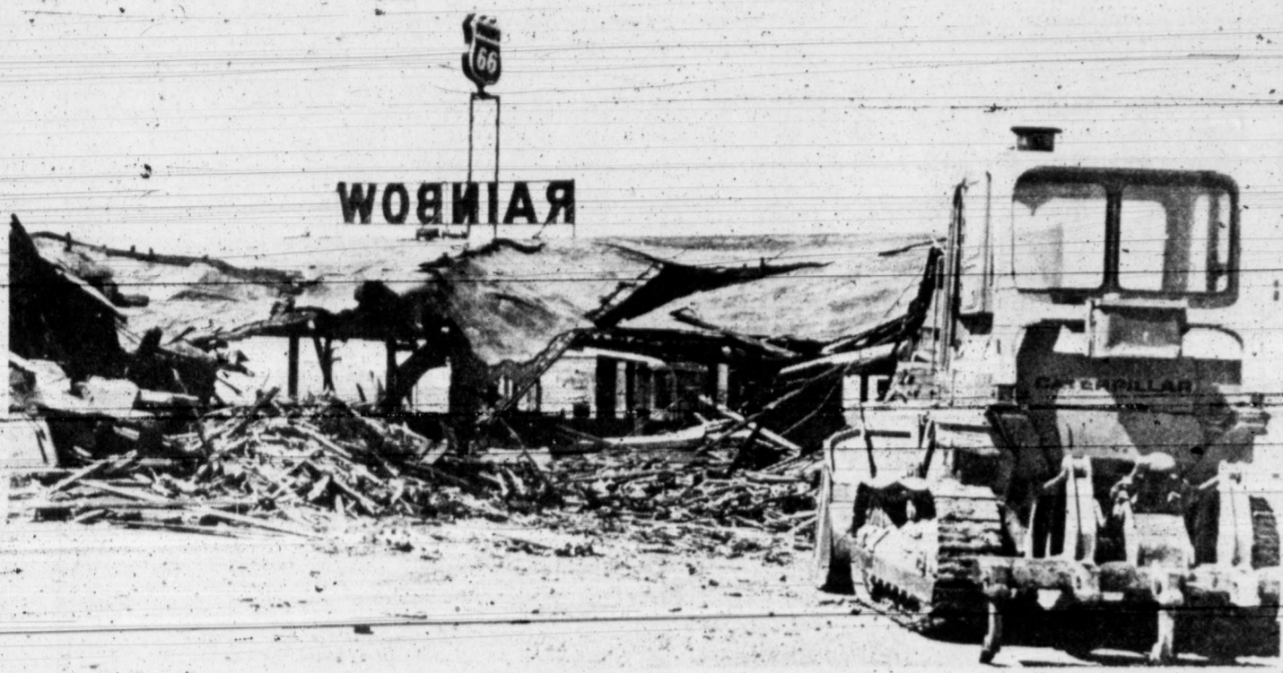
DEBRIS CLEARED—Debris was cleared Thursday from the site of the former Rainbow Market at 1614 25th St. The building and its contents were heavily damaged in a fire several weeks ago. (SDN Staff Photo)
