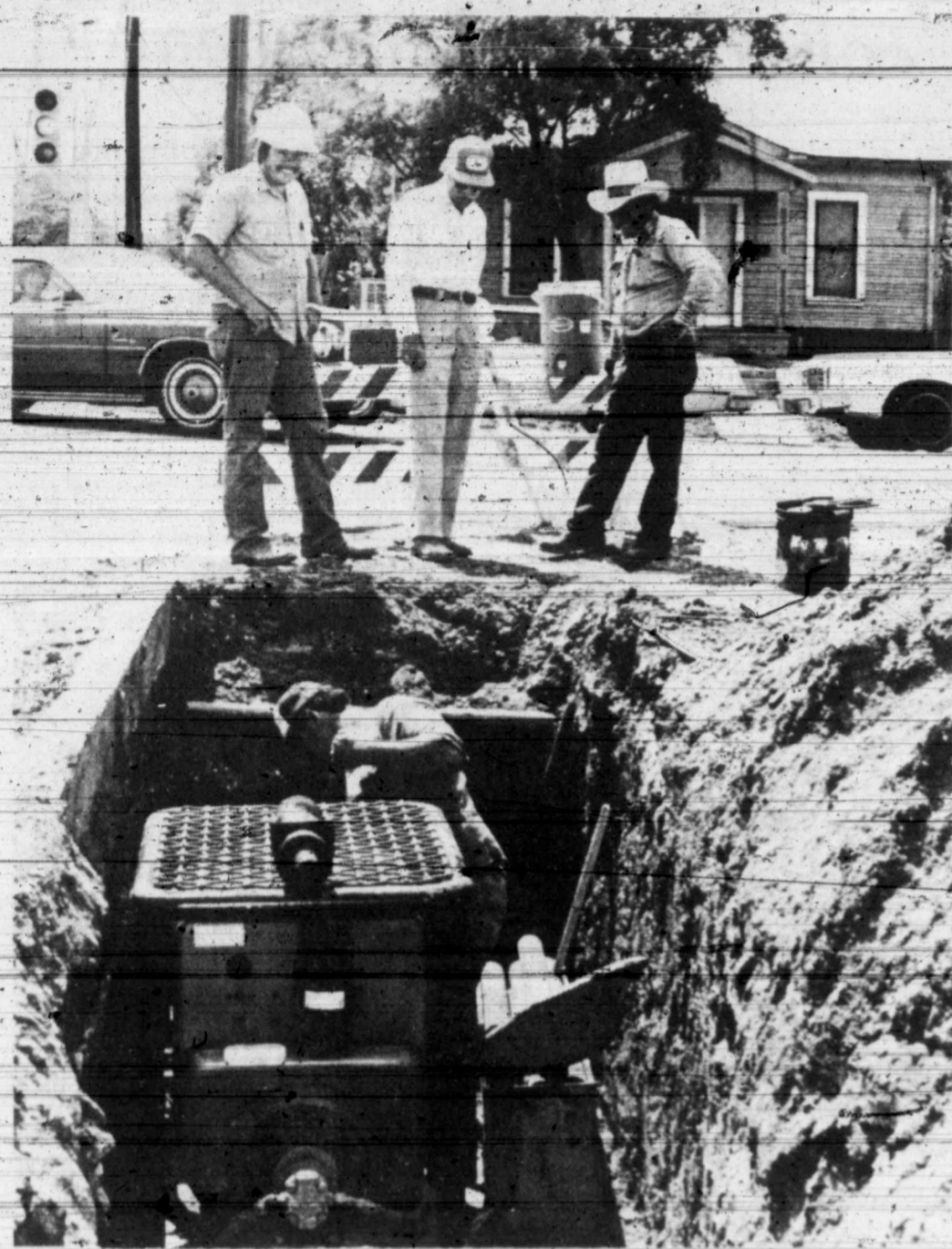
INSTALLING CONDUIT—Drilling and boring work has been initiated for the laying of telephone conduits for Southwestern Bell Telephone Co. The picture above was taken at 30th St. and College Ave. In the hole is Margarito Montez, working for Armadillo Boring of Odessa. Above the hole are, from left, Edward Stewart of Southwestern Bell, George Lee, city street superintendent, and Holiipo Cisneros, also representing Armadillo Boring Co. The conduits are being laid from the downtown telephone office to a point near the Towle Park entrance on College Ave. (SDN Staff Photo)
