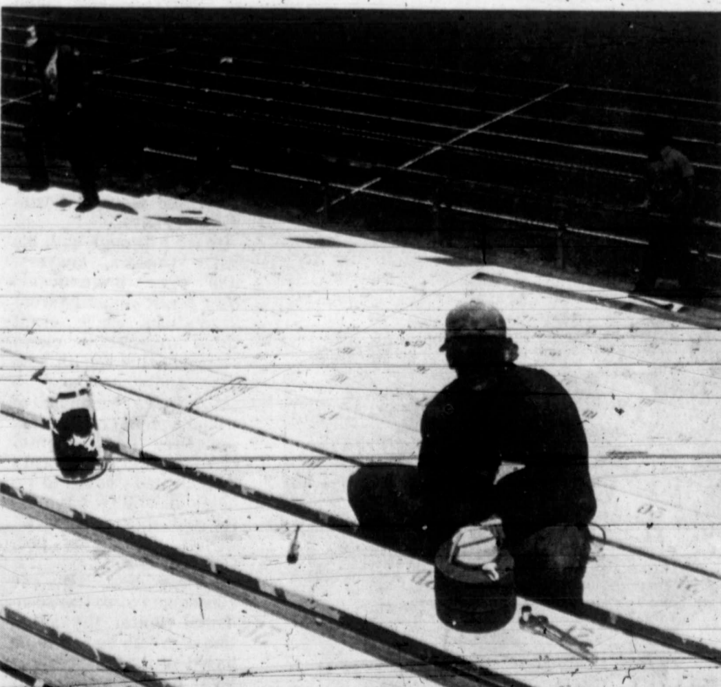
WALKWAYS REPLACED—Walkways on the west side of the bleachers at Tiger Stadium are being replaced. The work started about July 15 and is expected to be completed by Aug. 15. The boards are being replaced by aluminum planks. The work contract was awarded to Eddie Williams, a high school science teacher. In the photo above, George Adams saws through some wooden boards, while two assistants in the background prepare to throw an old wooden walkway board to the ground. (SDN Staff Photo)
