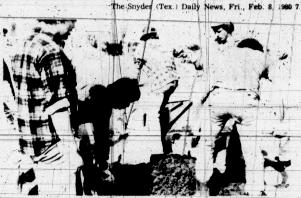
BACKBREAKING TASK —Rodney Hernandez of Snyder (dark shirt, white gloves) leans into the backbreaking task of mixing concrete by hand. He was part of a Hardin-Simmons University mission group that worked in El Sausal, Mexico, during semester break. (HSU Photo by Craig Bird)
