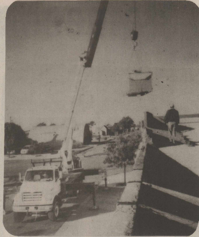
Mungia's set the heating/air conditioning unit, for the computer/reception area, Friday. The electrician will start working Monday, so things are moving right along.
