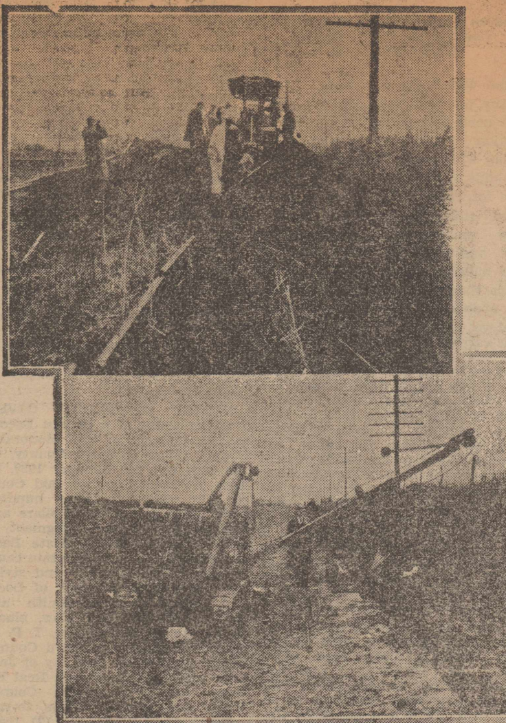
Upper—A specially built machine digging the three-foot trench for first underground long distance cable near Oklahoma City. Fiber conduit for cable is shown along side of trench. Lower—Back filler, filling in trench after conduit and cable is in place.
