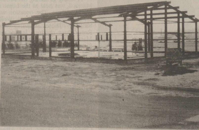
New Place--La Mision Bautista raising the roof on their new building at the corner of Wall and S. Fourth.
