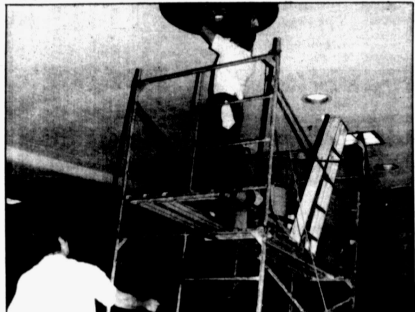
Ralph Contreras of Steamatic of the Permian Basin reinstalls a freshly cleaned vent in the Midland High School Auditorium. Larry Carlton helps steady the scaffolding.
