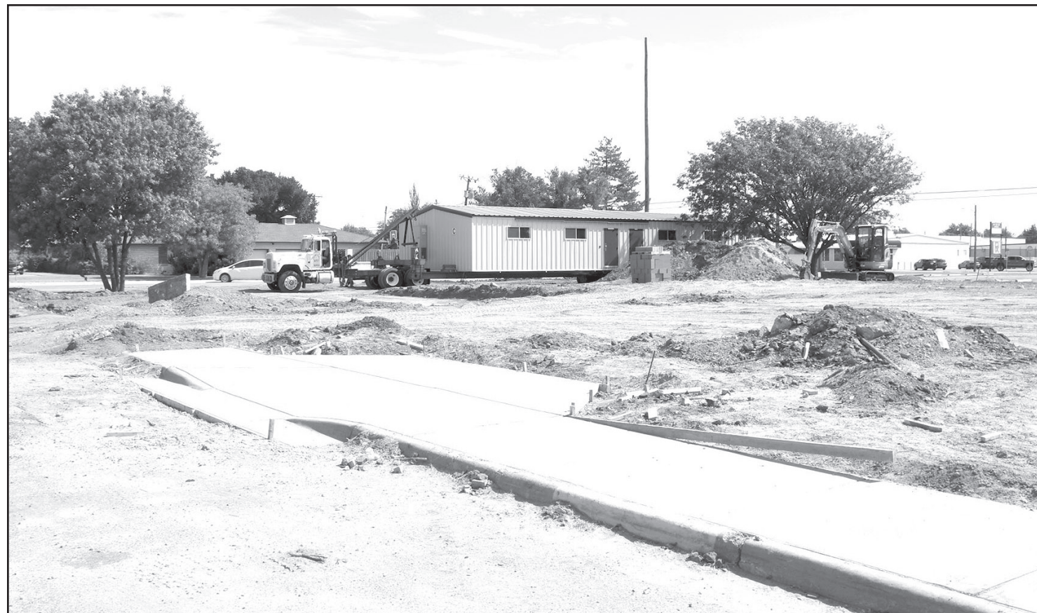
A portable building finds a new home at the north end of the old Primary School site. A second building will also be moved to its new home later in the week. In the foreground you can see part of a new sidewalk that was constructed on the west side of the lot. A new half-size football field and a parking area on the south end of the block will be installed in the next few weeks.
