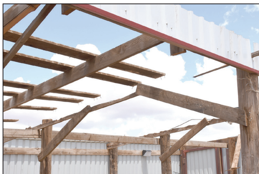
Part of the aftermath of Monday evening’s storm was roof damage at the FFA ag farm east of Friona. See other photos on back page.
