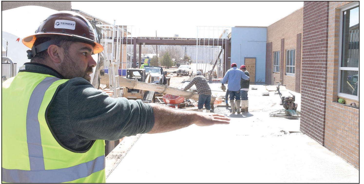
Superintendent Lorenzo Soto, of Teinert Construction directed a tour of the new Primary School for the Friona Noon Lions Club on Monday. Workers are pouring concrete on the east side of the new building on what used to be Cleveland Avenue. One of the corridors that will connect the new Primary School with the Elementary School can be seen in the background.
