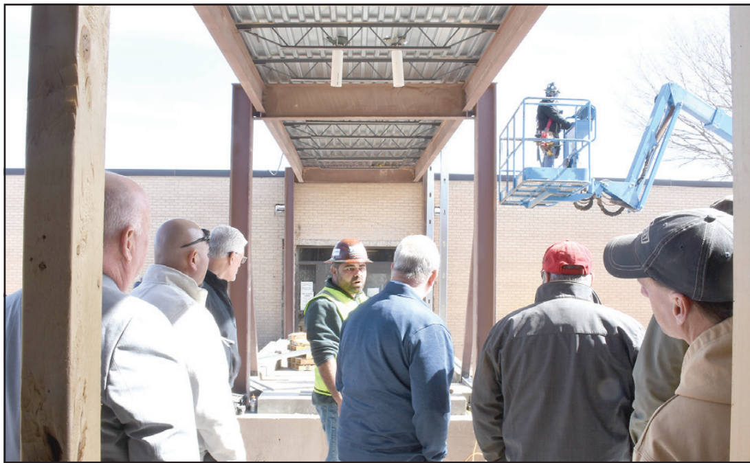
Lions Club members get a view of the north corridor that will connect the Elementary School with the new Primary School. Construction is on schedule with move-in set for late May. Exterior work and landscaping will continue into the Fall.
