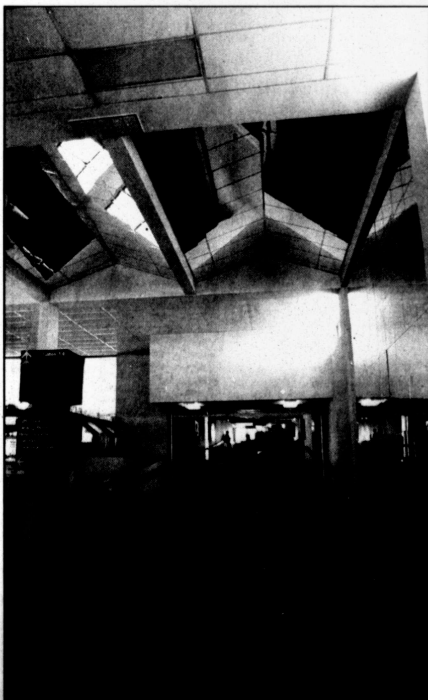
According to airport officials, there is asbestos insulation in the ceiling over the main walkway that leads to the concourse and in the ceiling above the ticket counters of the airlines.
