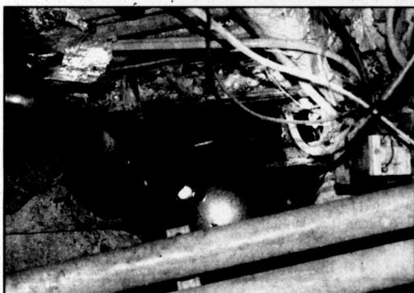
Water collects in this underground space where electrical connections and other pipes are located.
