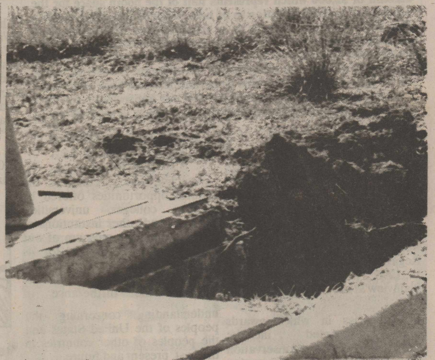
Stratford was without water on Wednesday, May 1 for approximately five to six hours because of a leak at the City Park. Shown above is a large hole that was at the park while it was being repaired. Stratford has lost Electricity, then water, WHATS NEXT?
