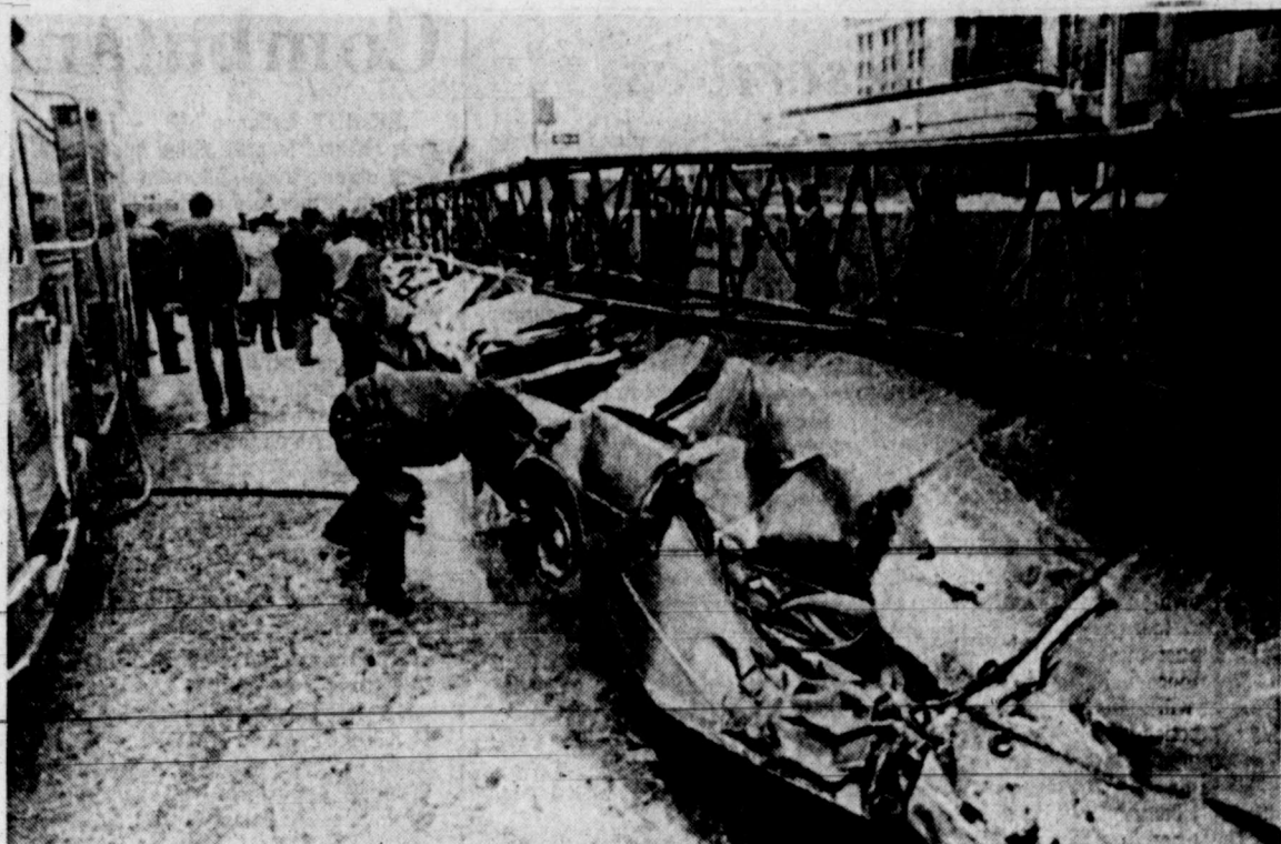
CRUNCH! — Seven cars, two of which were police cruisers, were damaged when a 300-foot-long crane toppled over while unloading steel at the site of the new Wayne County jail in Detroit. Four of the vehicles were parked in a no-standing zone when the crane inexplicably fell. Six persons were treated for minor injuries, but the crane operator, Ray Campbell, 62, was not injured during his abrupt trip sideways. The fine for parking in no-standing zones is normally $20 in Detroit. (AP Laserphoto)
