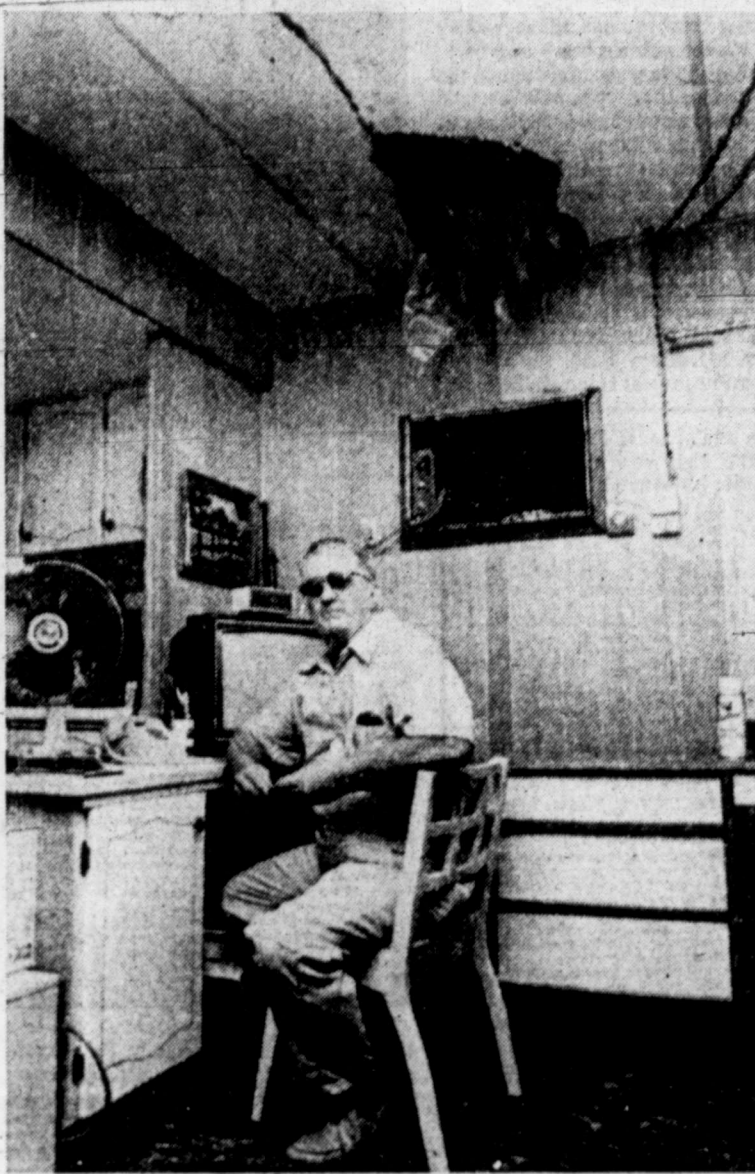
POT BOMBS HOUSE — Robert Banta sits by the hole in the ceiling of his mobile home in Fort Lauderdale, Fla., after a bale of marijuana smashed into it Thursday. The 100-pound bale was apparently dropped by a pot smuggler trying to evade customs officials at nearby Fort Lauderdale-Hollywood International Airport. After dumping an unknown number of bales, the airplane landed and the pilot escaped. (AP Laserphoto)
