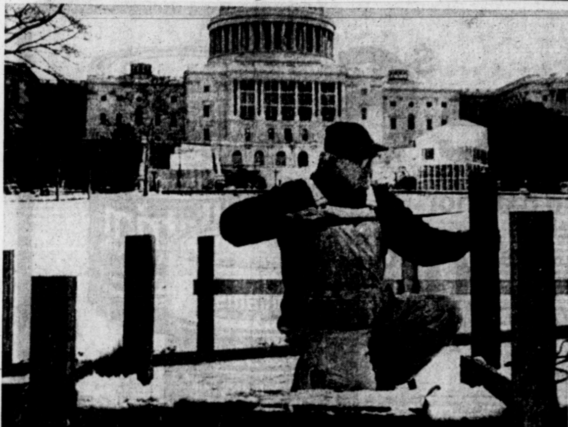
BUILDING INAUGURAL STAND — A workman puts his saw to work on stands that will be used on January 20 for the inauguration of President-elect Ronald Reagan. The west front of
